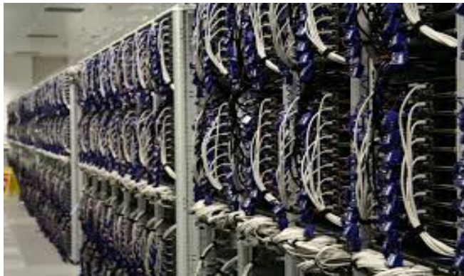
Data Center electrical Interconnect today
